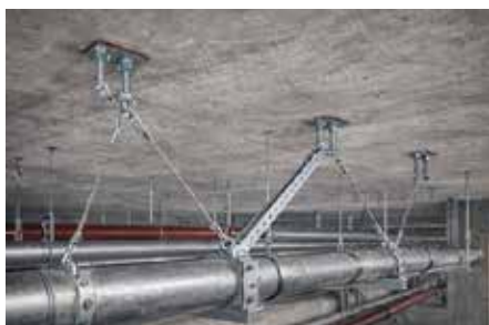
Pipe and ventilation systems
