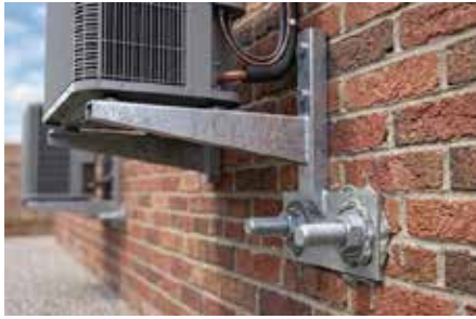
AC support on brick
